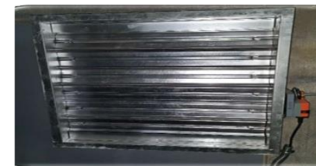
AUTOMATION OF AHU FRESH AIR DAMPER WRT. IAQ PARAMETERS
